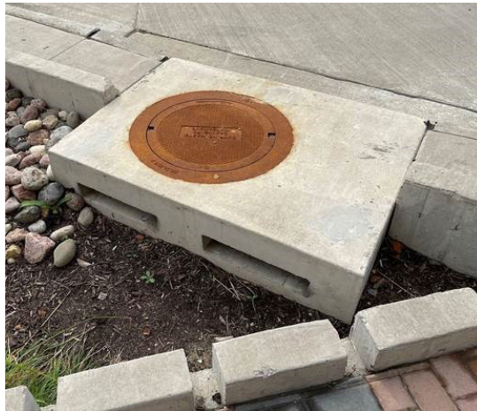
SUDAS Type SW-507 inlet modified to include a sump, with two small openings that overflow into the planter box in Coralville, Iowa.
