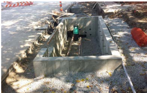
An overflow inlet shown during construction in a planter box in Coralville. The small holes in the side of the box allow for subsurface water movement into adjacent subsurface rock chambers.
