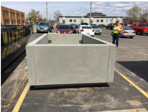
Precast mockup of planter boxes to test methods of assembly for those to be installed in La Crosse, Wisconsin.
