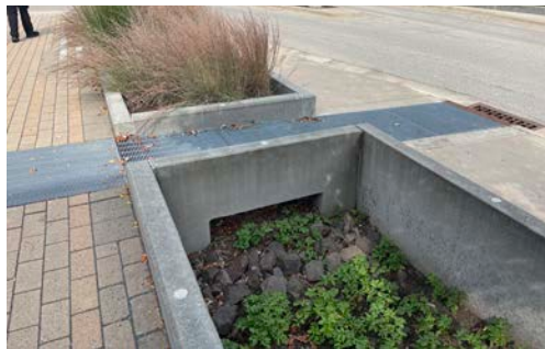
In this location, the inlet itself acts as an overflow. Once the planter box is full of water to the gutter elevation, water will continue downstream to the next storm inlet (in La Crosse, WI).
