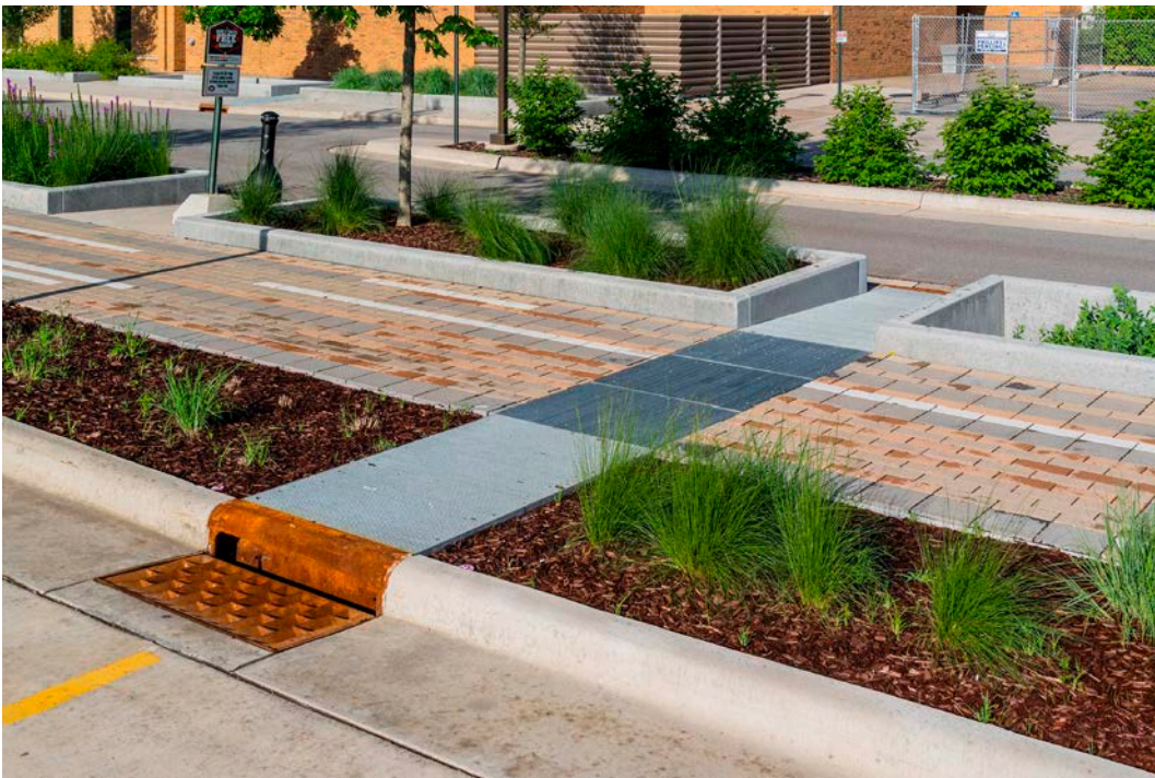
A concrete flume below a metal gate connects two sump inlets to the stormwater planter box in La Crosse, Wisconsin. For record drawings, the information listed above would need to be surveyed.
