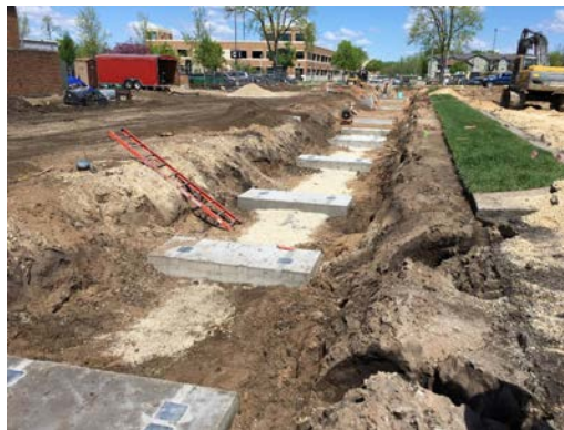
Precast foundation units placed prior to installation of precast planter boxes to be installed in La Crosse, Wisconsin.
