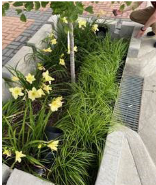
A small concrete sump is located under the small grate at the curb cut in this photo in Coralville, Iowa.
