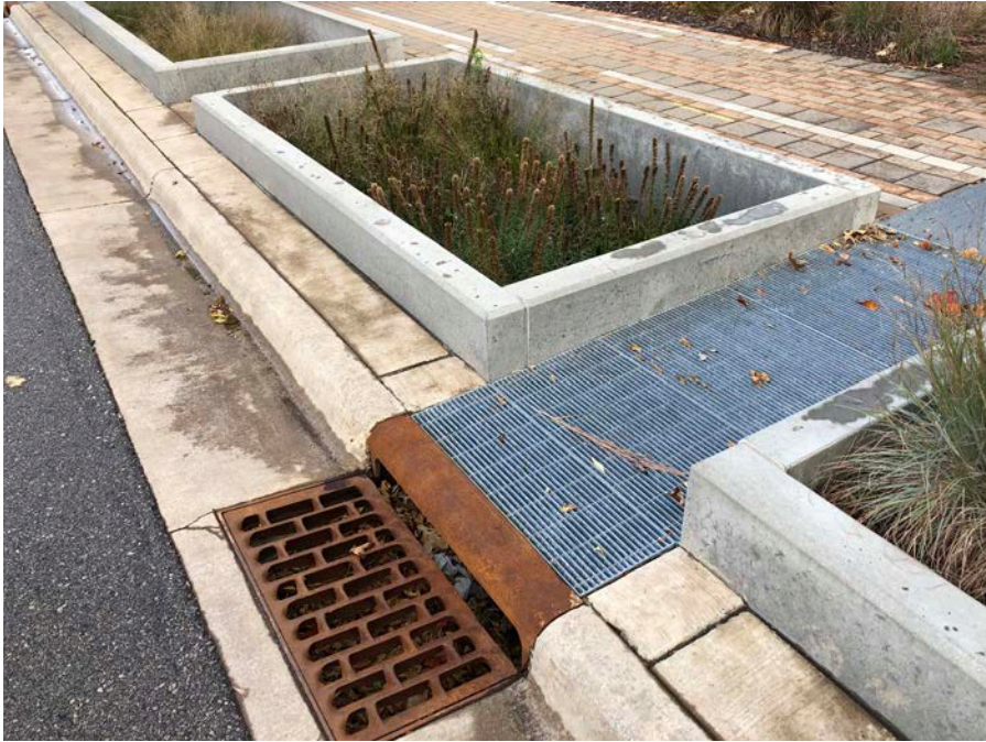
This photo was taken in La Crosse, Wisconsin in September, five years after installation. Fall leaves have collected in the sump and need to be removed.
