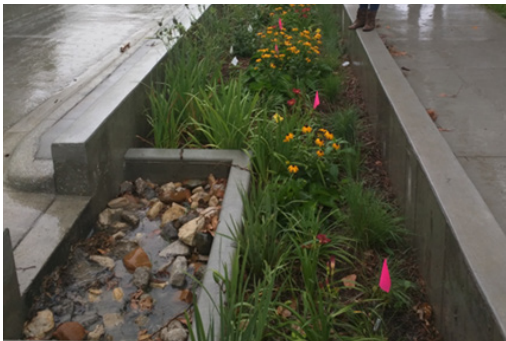
Curb cut entry from street into stormwater planter in Coralville, Iowa.
