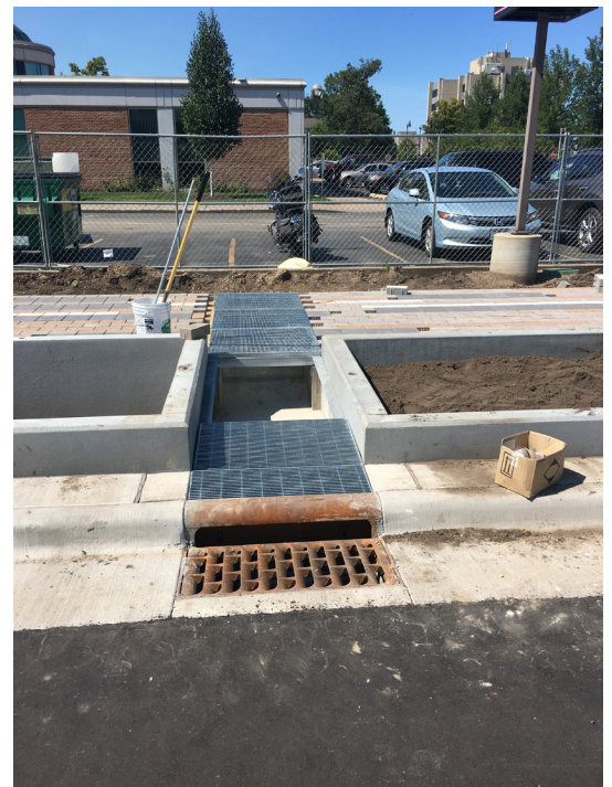
Construction of overflow flume from catch basin sump to planter boxes in La Crosse, Wisconsin.
