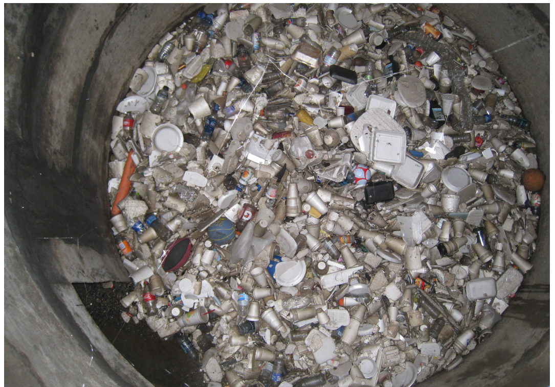
Trash collection inside an HDS unit.
