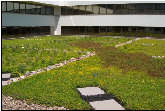
(c) A 4,700 square foot modular extensive green roof installed at Genesis Medical Center in Davenport in 2010.
