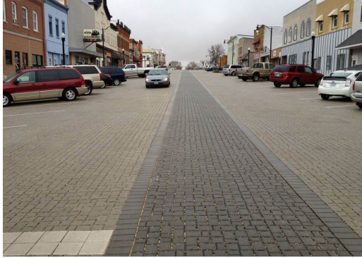
FIGURE C8-SU-1: Example of permeable pavement system in West Union, Iowa.
