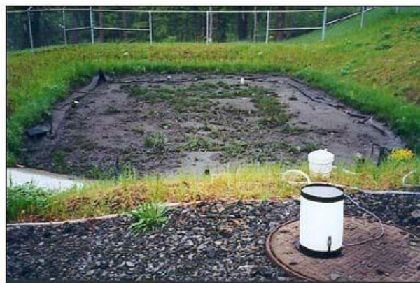
Figure C6-S1- 5: Surface sand filter
