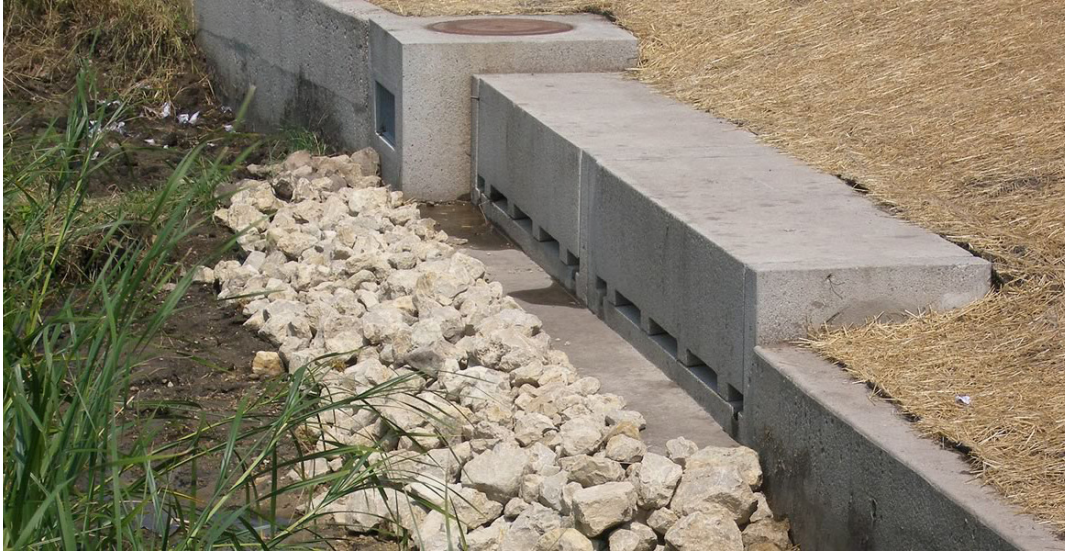
Level spreader outlet structure at Heritage Park in Minneapolis, MN. (photo courtesy - Mississippi Watershed Management Organization mwm.org )
