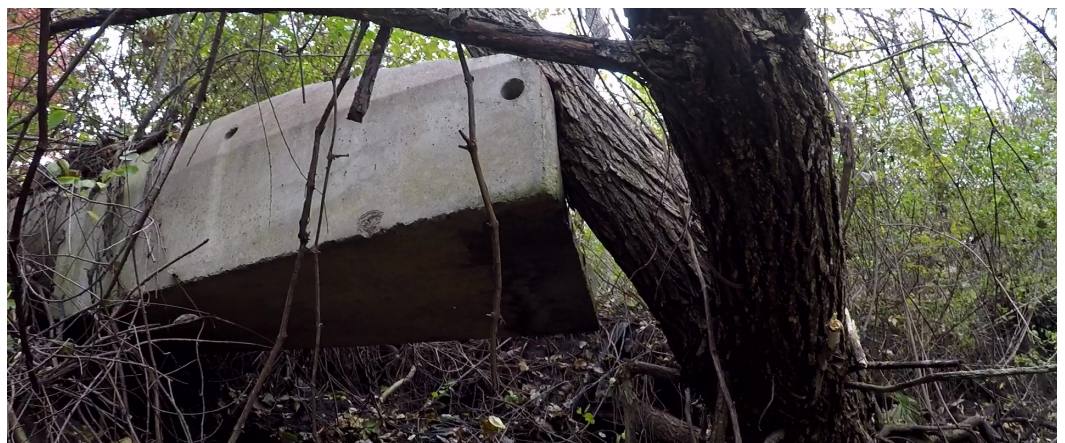
Figure 9.11-1-14: Unstable outfall photo
