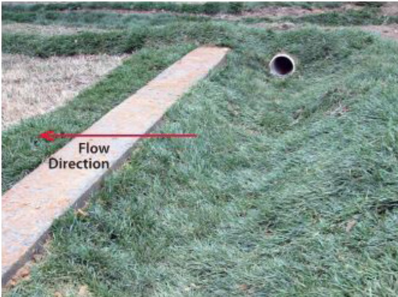
Concrete level spreader with grass basin on upstream side. Flow enters from pipe that runs parallel to the spreader and leaves by filling the basin and flowing across the level concrete strip. (photo courtesy - NC State University "Urban Waterways - Level Spreader Update")
