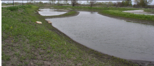
The berms and depressions of microtopography can be seen as the wetland fills just after construction.
