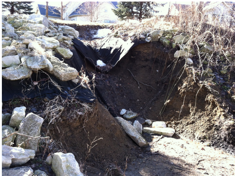
Photo 9.01-1-2: Bank erosion caused by detention basin frequently overtopping
