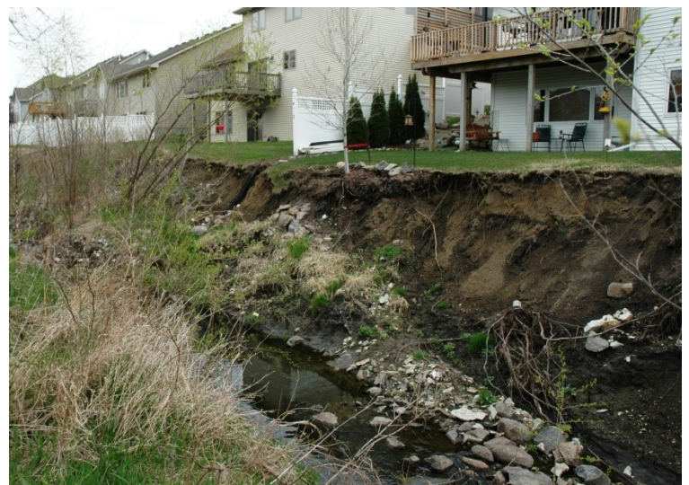
Photo 9.01-1-1: Example of Streambank and Channel Erosion caused by hydrologic changes in an urbanizing area in Central Iowa
