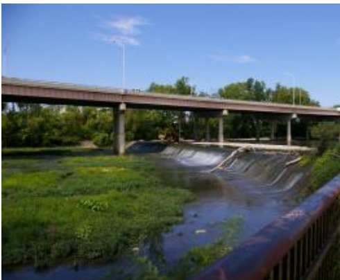
Photo 5. Pre-construction view of 5 th Avenue Dam on the Olentangy River in Columbus, OH. Source: Stantec.
