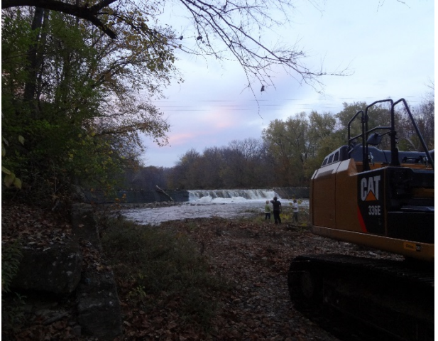
Photo 7. First notch placed in West Milton Dam during phased removal. Source: Stantec.
