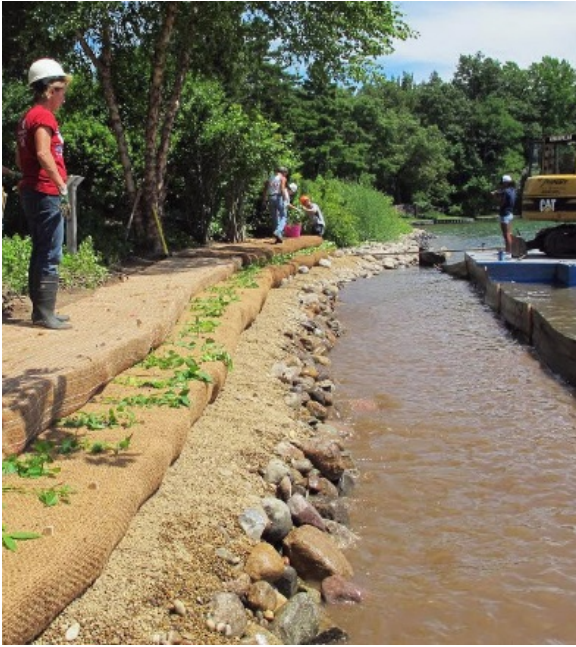
Photo 8. Construction of bank with fabric encapsulated soil lifts over stone toe protection. Source: Michigan State University Extension.
