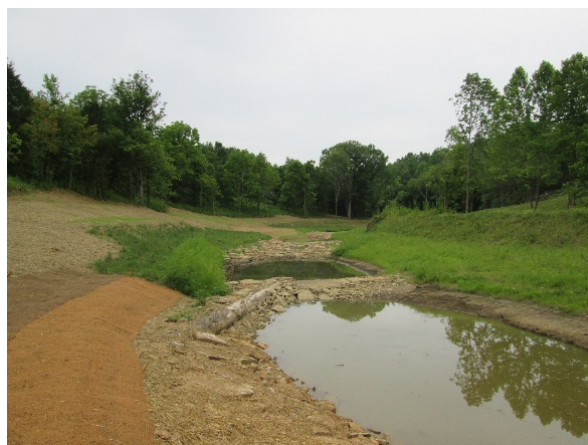
Photo 13. Newly constructed log vane with boulder hook on Minors Creek. Source: Stantec.
