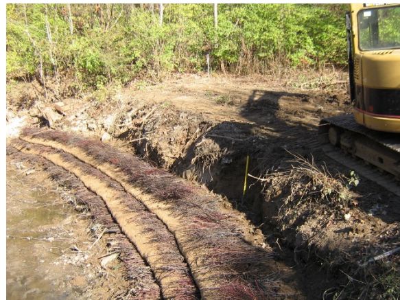
Photo 11. Construction of soil lifts with live brush layering at Cherokee Park. Source: Stantec.
