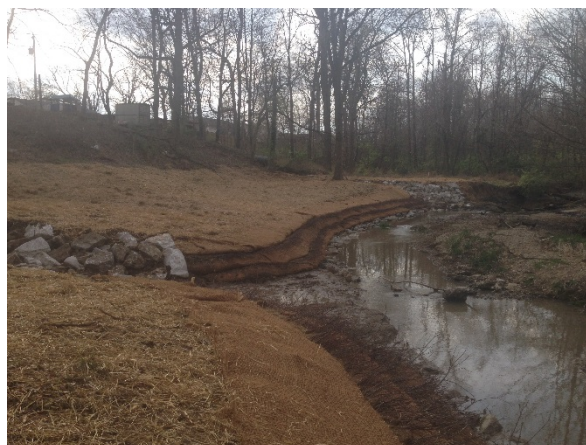
Photo 6. Construction of bank with stone toe protection and soil wraps with live brush layering. Source: Stantec.
