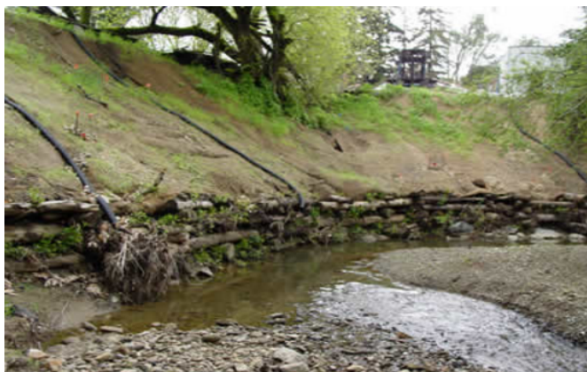
Photo 10. Submerged Cribwall. Source: Unknown.
