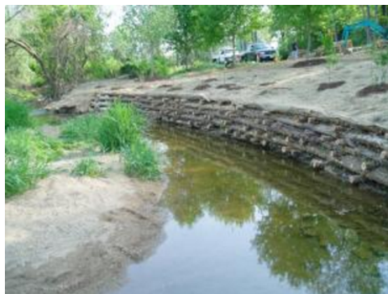
Photo 4. Submerged Crib Wall. Source: Unknown.
