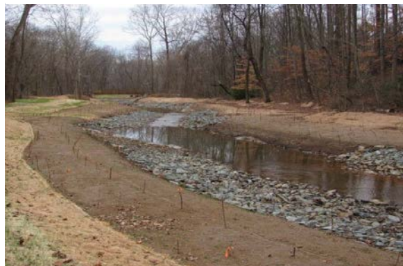
Photo 4. Example 2 - Stream banks after reshaping and armoring. Source: The Nature Conservancy & City of Charlottesville
