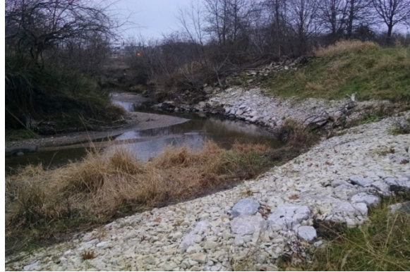
Photo 2. Example 1 - Jordan Creek after bank shaping with rock toe protection. Source: LT Leon Associates
