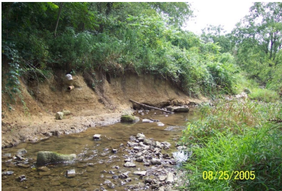
Photo 9. Big Cove Creek prior to bench construction. Source: Fulton County Conservation District
