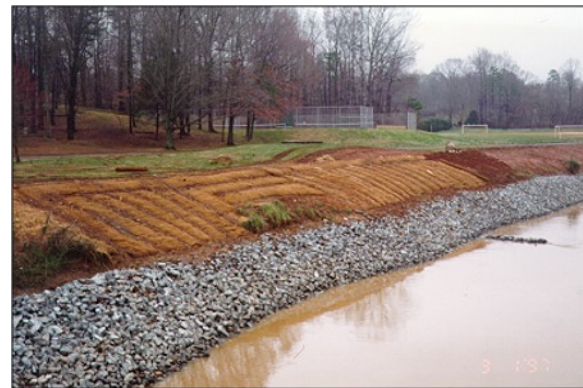
Photo 16. Fascines placed at angles and on contours. Source: Charlotte-Mecklenburg Storm Water Services
