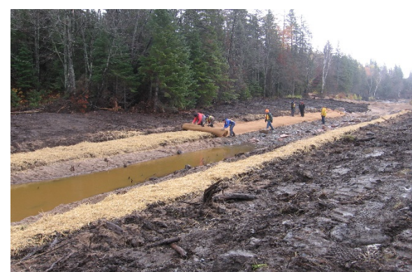
Photo 30. Erosion control matting being rolled onto a stream bank. Source: Collins & Baker Engineering
