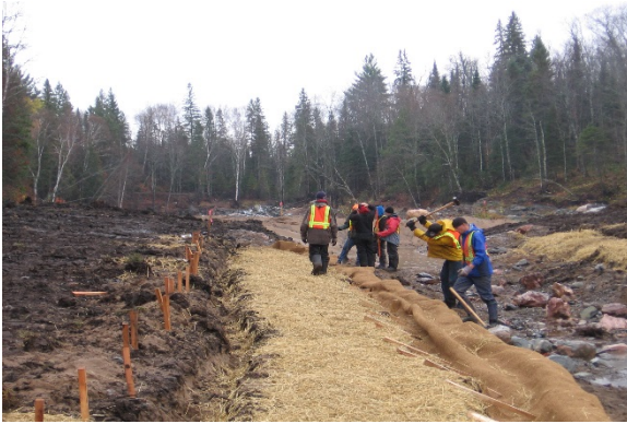
Photo 25. Top of slope trench for erosion control matting anchor. Source: Collins & Baker Engineering
