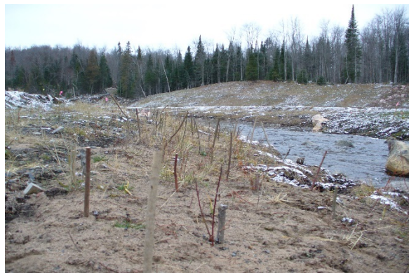
Photo 12. Live stakes installed in late autumn on Dead River, MI. Source: Collins & Baker Engineering
