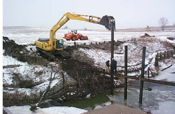
Photo 30. Sheetpile being driven for Grouted Grade Control Structure. Source: Hungry Canyons Alliance.
