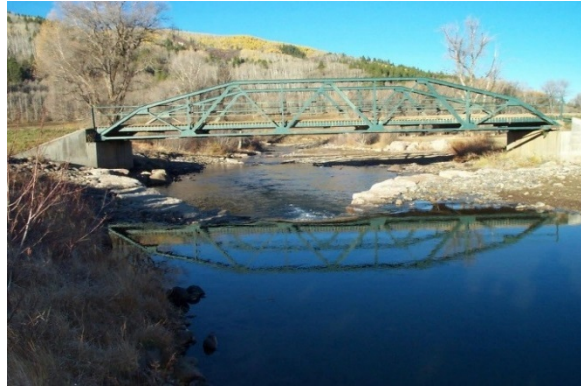
Photo 6. Cross vane arms tying in to bridge abutments. Source: Blue River, Wildland Hydrology.
