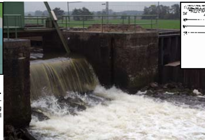
Floating slide. Recirculation eliminated with floating slide in a Dutch canal
