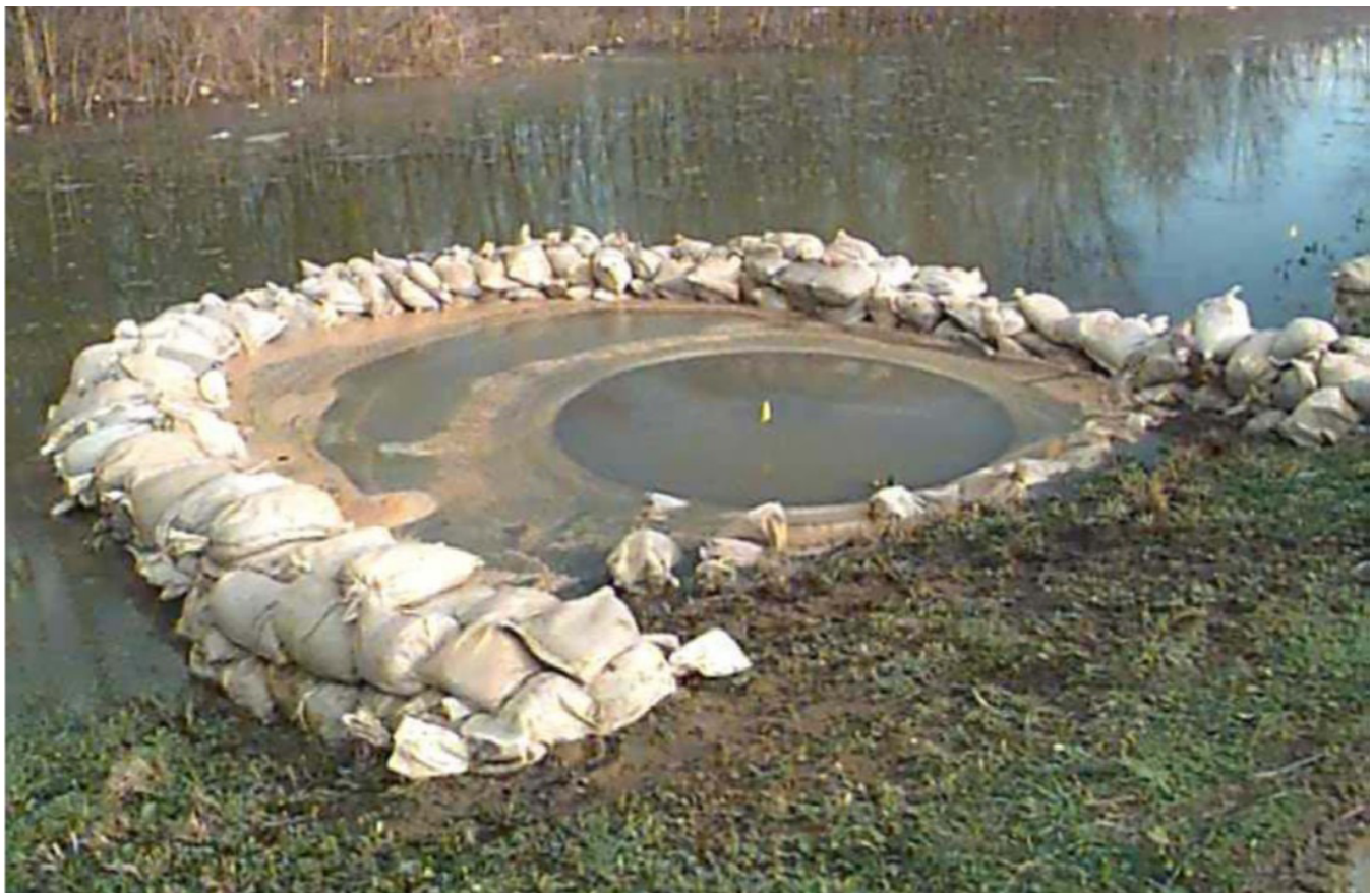
Figure 20: Sandbag Ring Levee around a Boil at the Downstream Toe of an Embankment Dam
