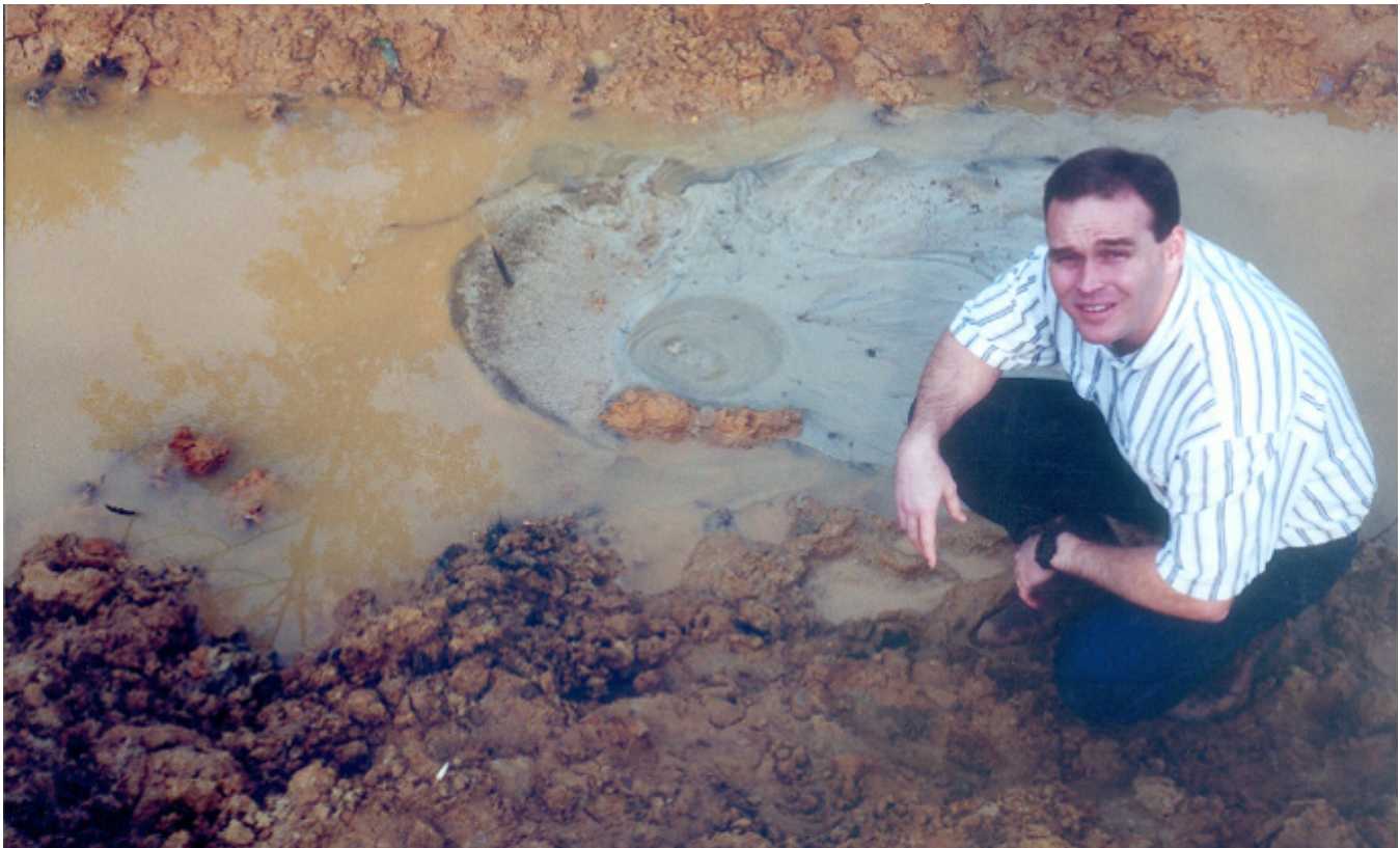
Figure 5: Boil at the Toe of an Embankment Dam
