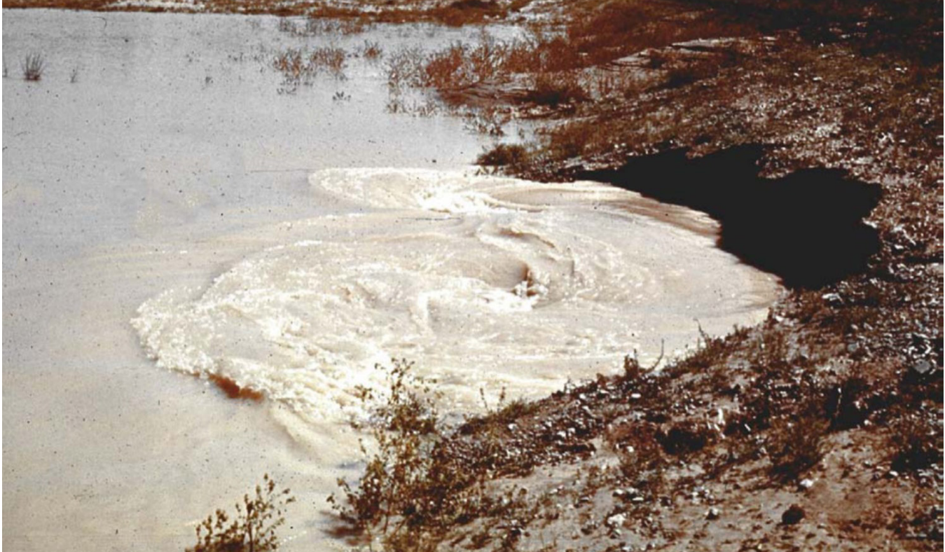
Figure 7: Photo of a Whirlpool at the Upstream Slope of an Embankment Dam
