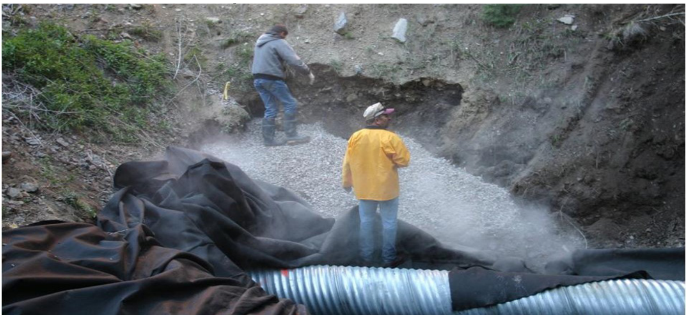
Figure 26: Example of Filter Diaphragm Construction around a Conduit in an Embankment Dam
