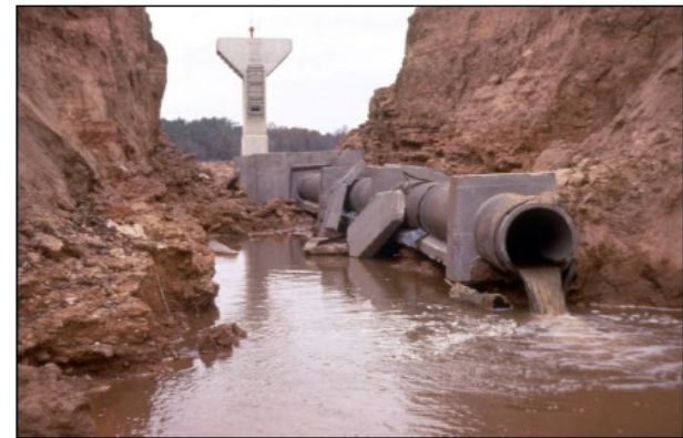
Figure 2-5. Embankment dam breached after piping along the conduit. The view is upstream. Note pre-cast concrete pipe placed on a concrete cradle and the use of seepage collars (Photo credit NRCS).
