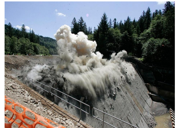
Marmot Dam, Sandy River, Oregon
