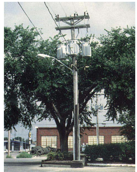
Figure 2. Grown into a power pole.
