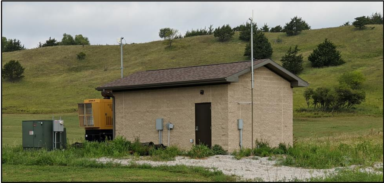
Well house with emergency generator
