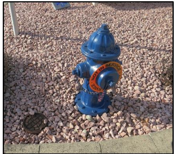
New hydrant, not yet in service
