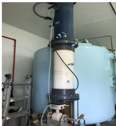
Pilot project for ammonia removal
