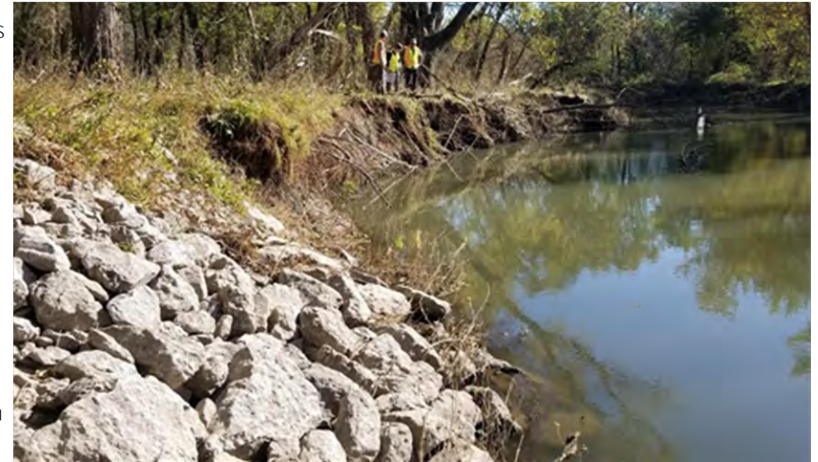
Figure 4-5. Large rip rap armoring a bank with instability immediately downstream
