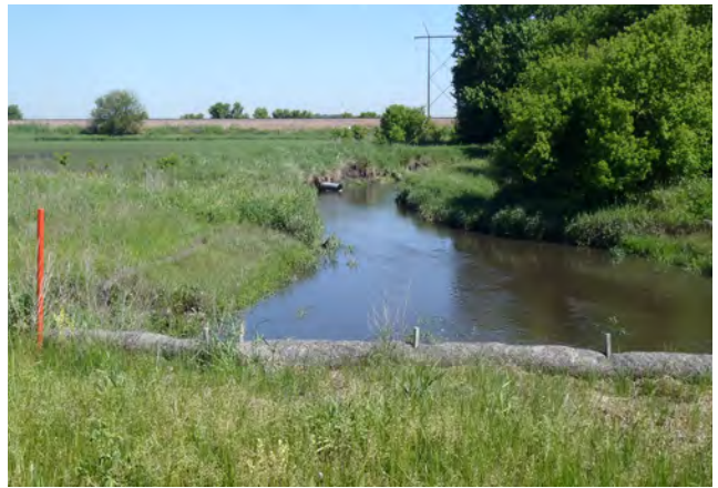
Bank movement has left this tile outlet projecting into the stream in the Beaver Creek watershed.
