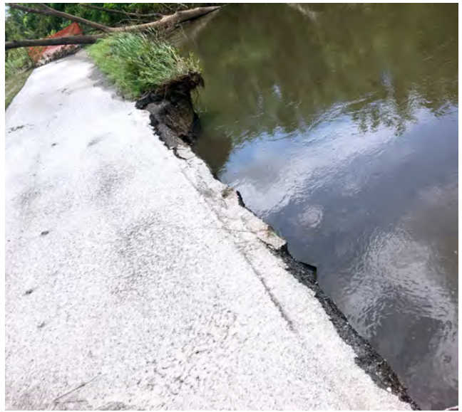
Bank erosion near a public trail (City of Johnston).
