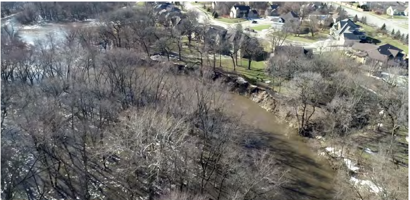
Aerial image of an unstable streambank (City of Johnston).
