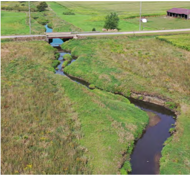
Bank erosion along a tributary to Beaver Creek.
