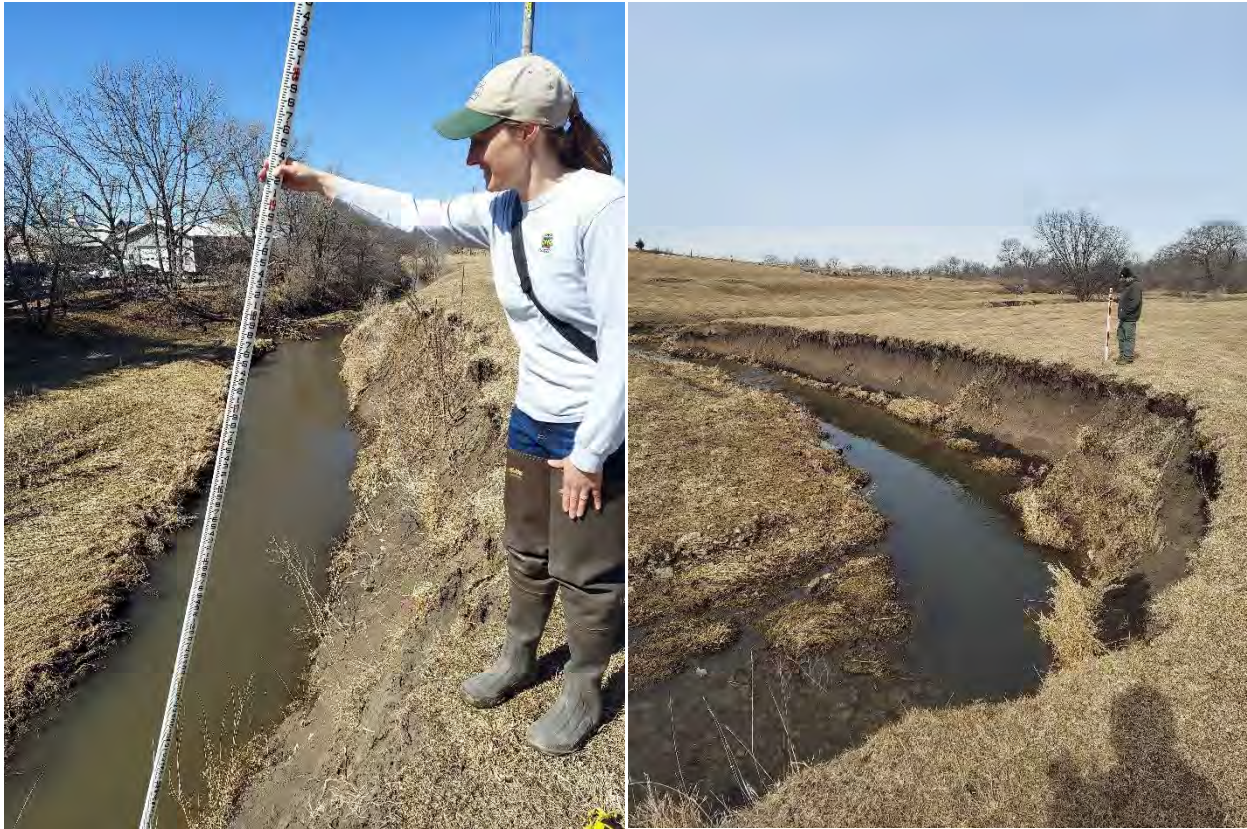
Figure 31. Moderate to severely eroded stream banks observed and measured during a RASCAL stream survey in the Trout Run Watershed.
