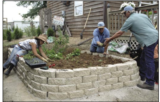
A retaining wall was installed to create a level rain garden on this sloping site in Madison County.
