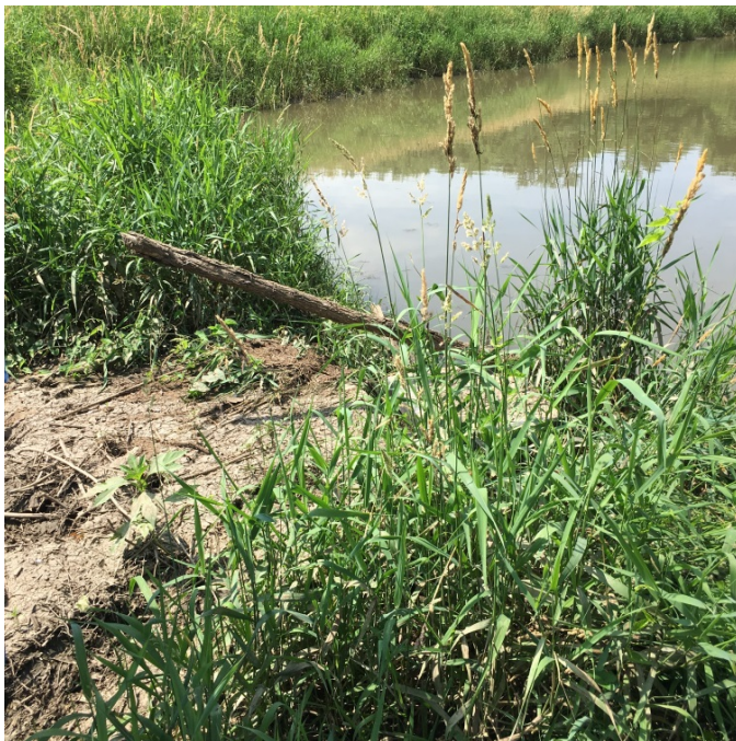
Figure 7. Broken culvert at outlet of silt pond.
