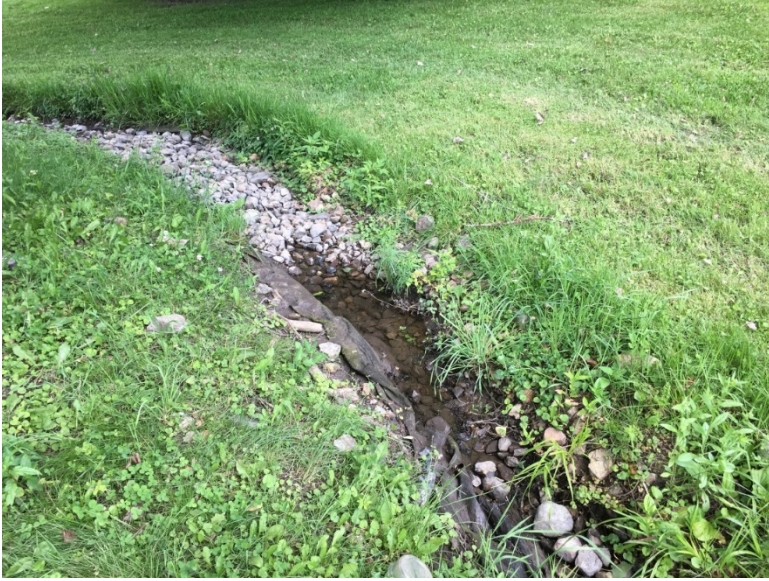
Figure 2. Poor condition of waterway / ditch draining along north side of beach.
