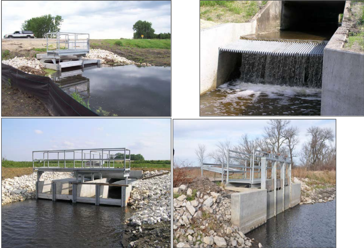
Photo: Water Control and Fish Barriers installed in 2011.
