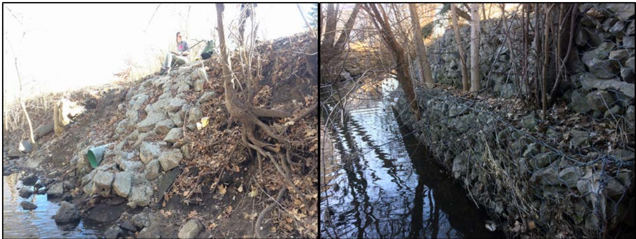
Figure 42. The image on the left shows a poor example of bank stabilization, where debris and cement was slopped into the stream and down the bank. Concrete is not a good way to stabilize it gives no movement for the stream and will speed up the waters movement causing more erosion to occur. The image on the left is between UNI's campus and College Street where apartments are being built, these apartments are right on the streams edge and rip rap was implemented to control bank erosion throughout this area. This kind of stabilization will help to prevent erosion, but not allow the steam to move at all.
