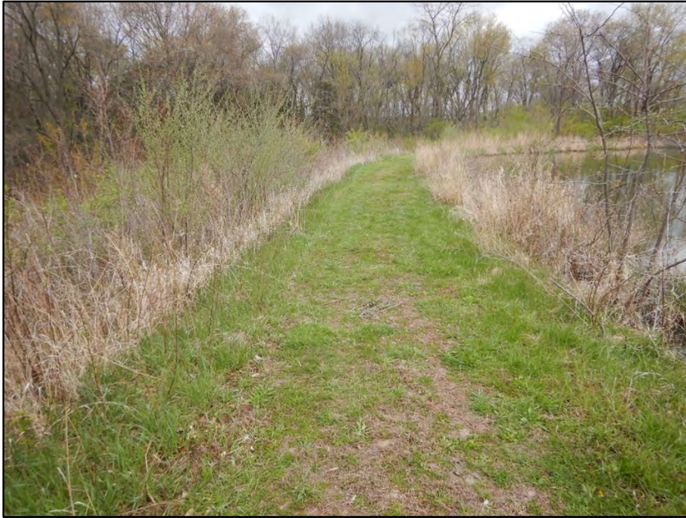
Figure 1: Photo taken on 4/20/21 showing the dam alignment with trees and brush growing on upstream and downstream slopes.
