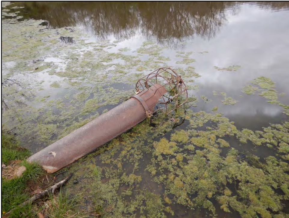
Figure 22: Photo taken on 4/20/21 showing the principal spillway with hooded inlet and rebar trash rack.
