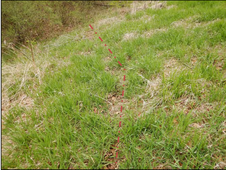
Figure 37: Photo taken on 4/20/21 showing possible microslide signified by line of bare earth 2/3rds up the downstream slope of the dam.
