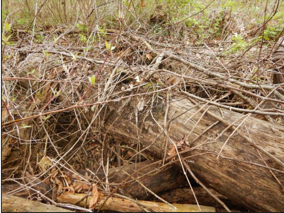
Figure 5: Photo taken on 4/20/21 showing debris surrounding the spillway outlet.
