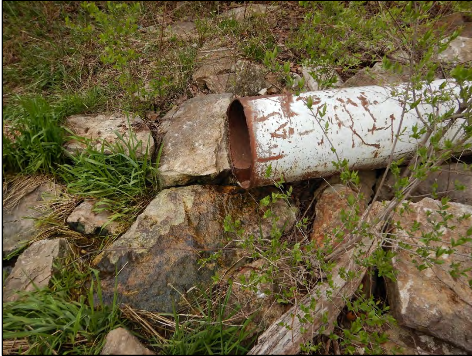
Figure 35: Photo taken on 4/20/21 showing the principal spillway outlet.
