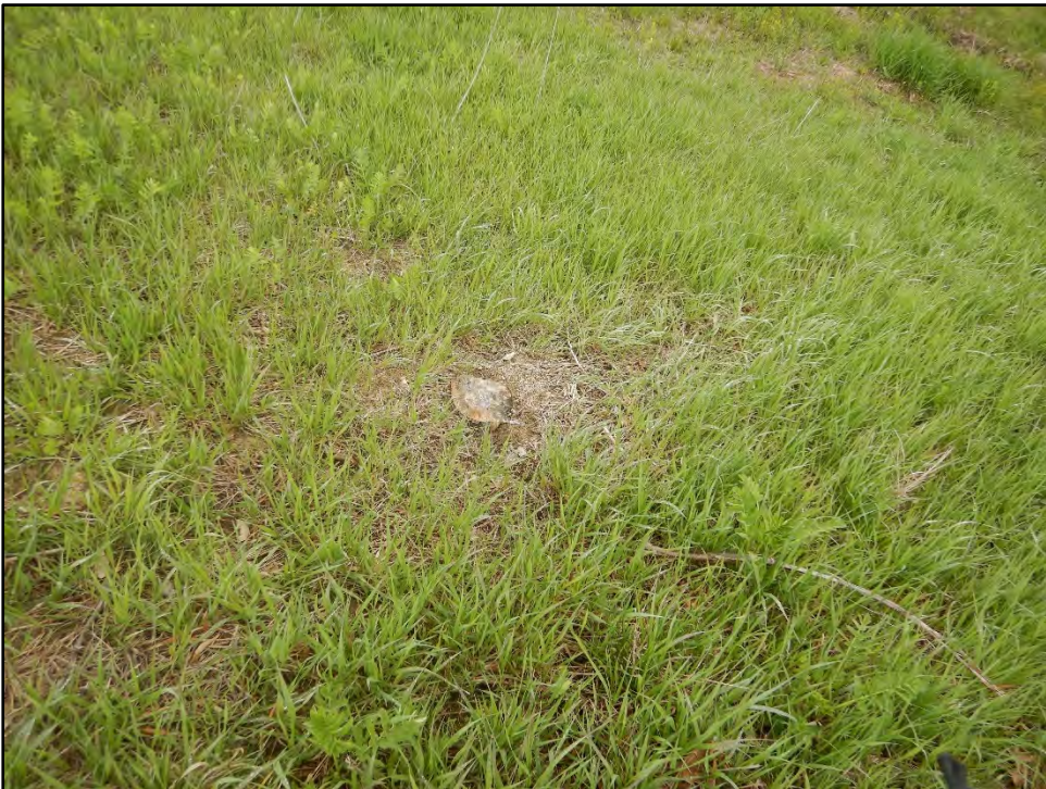
Figure 28: Photo taken on 4/20/21 showing a stump from cut tree on downstream slope of the dam.
