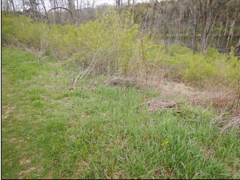
Figure 49: Photo taken on 4/20/21 showing large amounts of trees and brush on the downstream slope of the dam.
