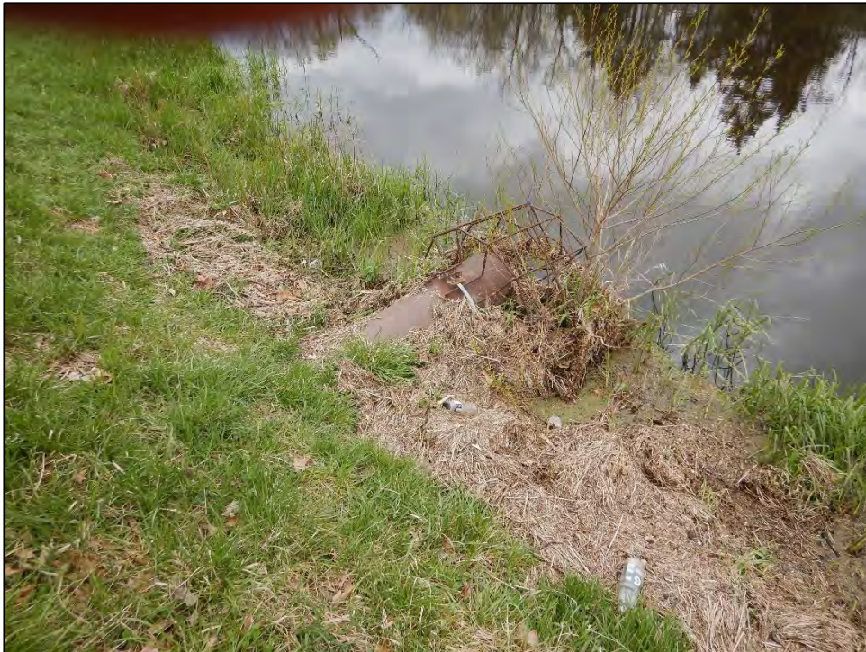
Figure 34: Photo taken on 4/20/21 showing the 18" diameter steel principal spillway inlet pipe with rebar trash rack and minor brush growing around inlet.
