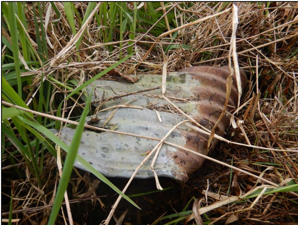
Figure 44: Photo taken on 4/20/21 showing the bent 6" CMP principal spillway inlet.
