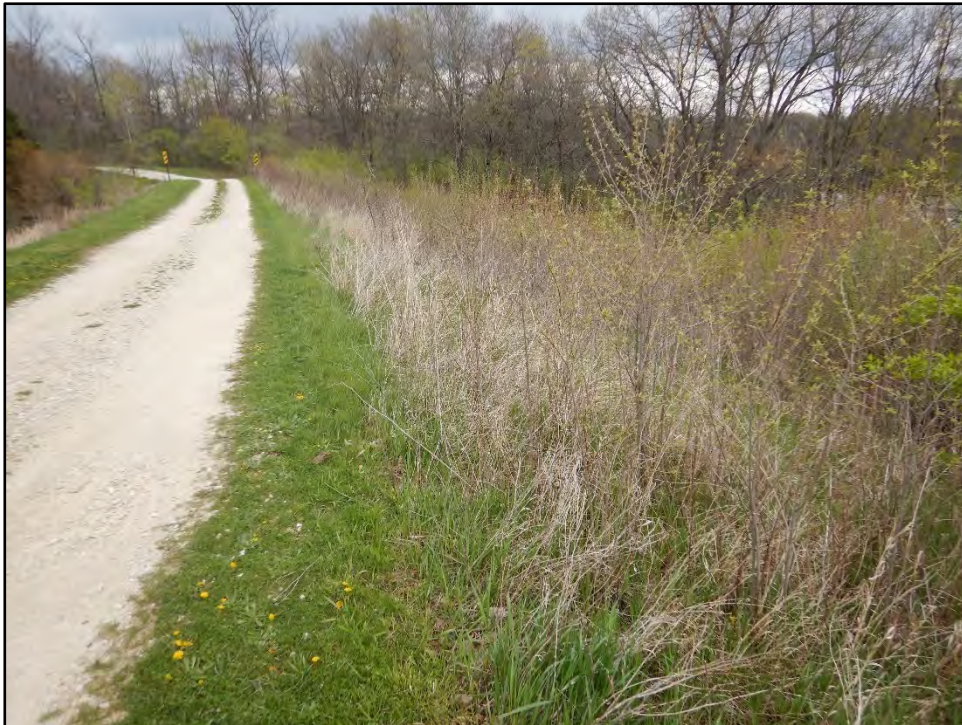
Figure 42: Photo taken on 4/20/21 showing the large amounts of trees and brush growing on downstream slope of the dam.
