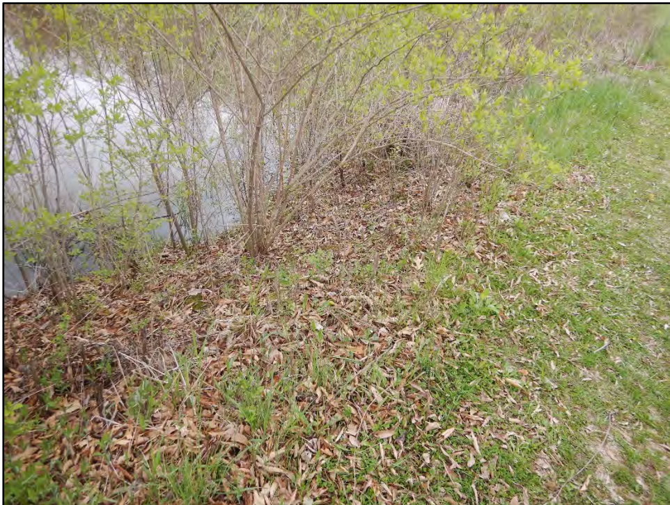
Figure 48: Photo taken on 4/20/21 showing the upstream slope and a few trees and brush growing at the water line.
