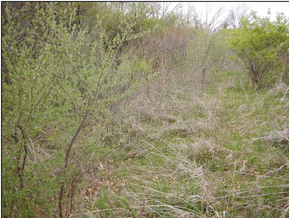
Figure 46: Photo taken on 4/20/21 showing the large amount of brush on the downstream slope of the dam.
