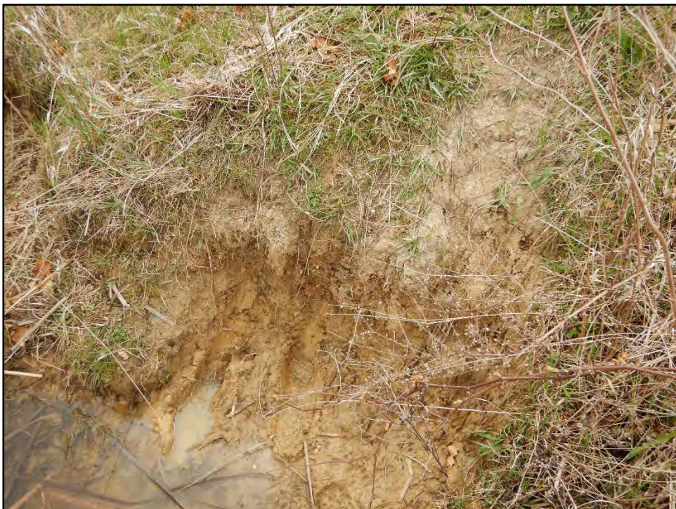
Figure 14: Photo taken on 4/20/21 showing minor erosion at water line.
