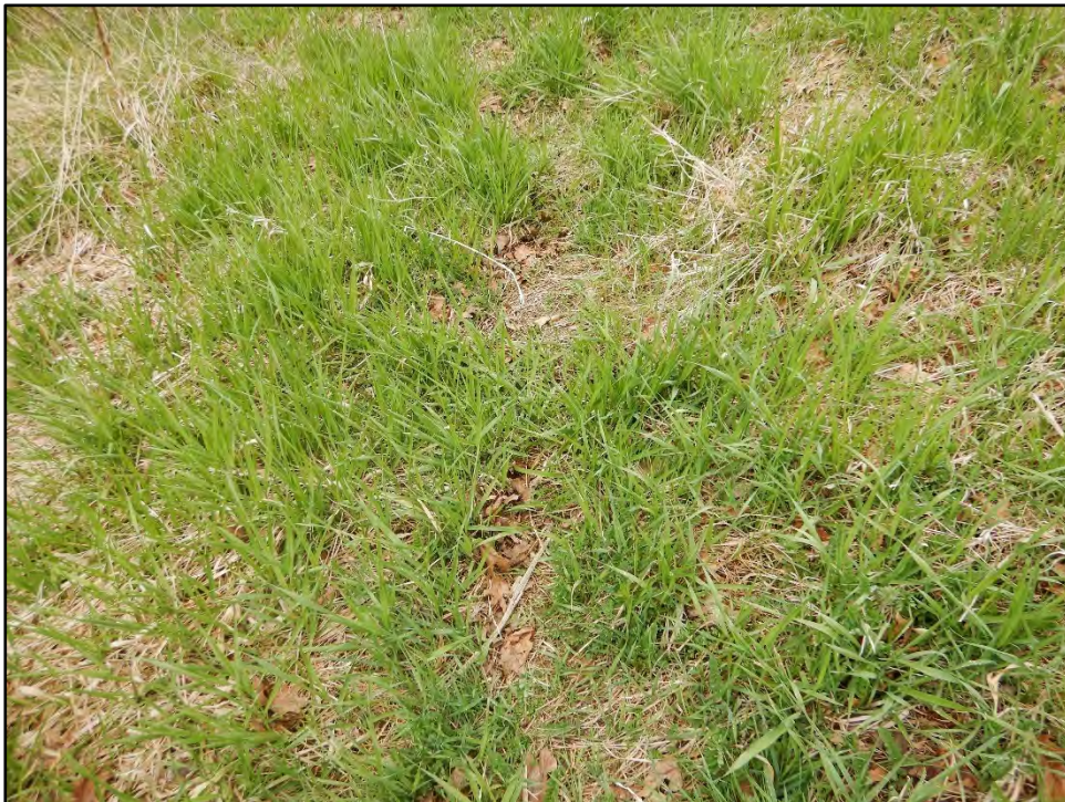
Figure 38: Photo taken on 4/20/21 showing possible microslide signified by line of bare earth 2/3rds up the downstream slope of the dam.
