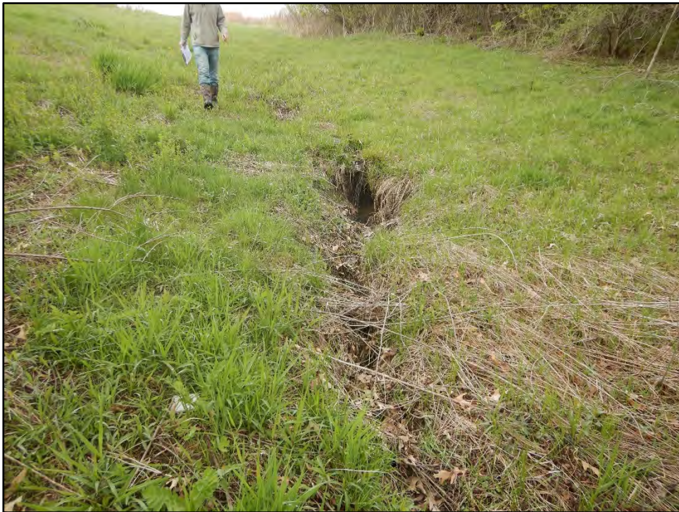
Figure 26: Photo taken on 4/20/21 showing minor erosion from local drainage along the groin of the downstream slope.
