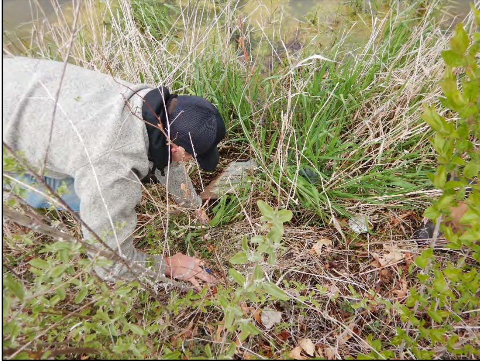
Figure 43: Photo taken on 4/20/21 showing the principal spillway inlet with brush growing around the inlet.
