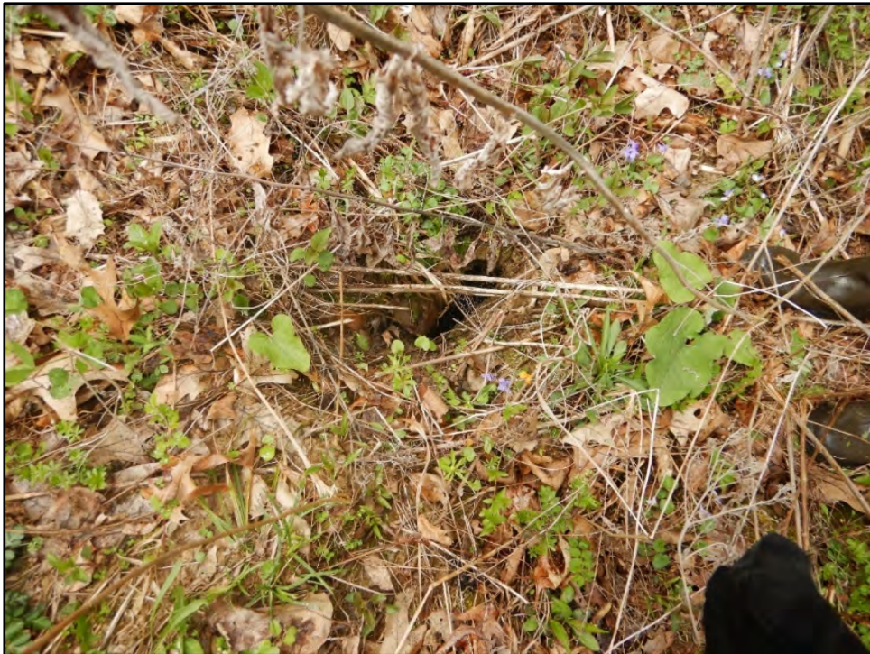
Figure 8: Photo taken on 4/20/21 showing seepage hole with running water along the principal spillway alignment.
