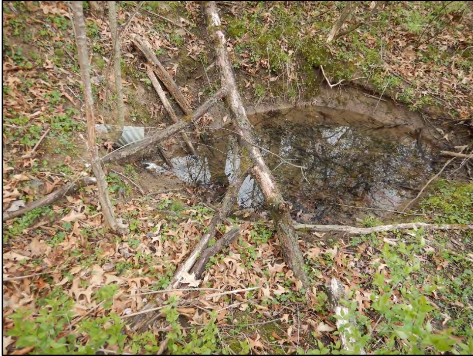
Figure 45: Photo taken on 4/20/21 showing 6" CMP principal spillway outlet with small scour hole.
