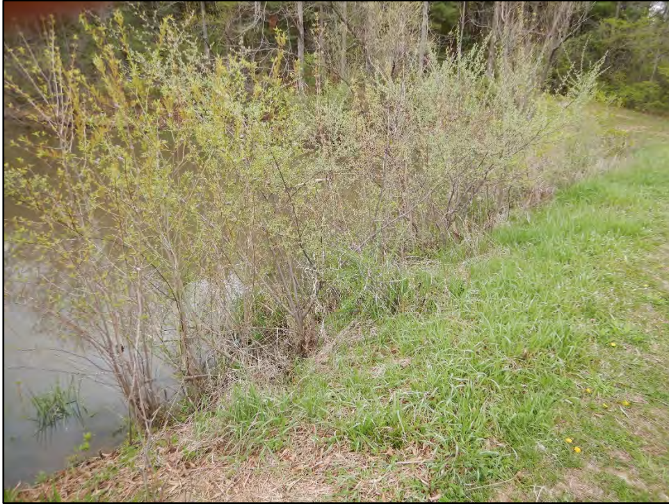
Figure 51: Photo taken on 4/20/21 showing some trees and brush growing at the water line on the upstream slope.
