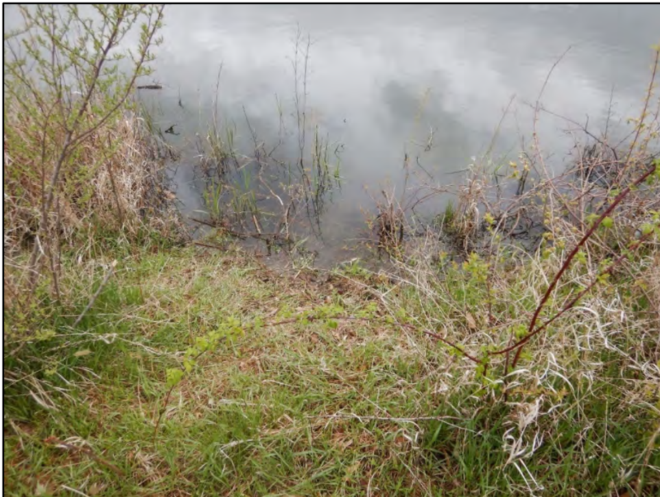
Figure 4: Photo taken on 4/20/21 at approximate location of the submerged principal spillway inlet.
