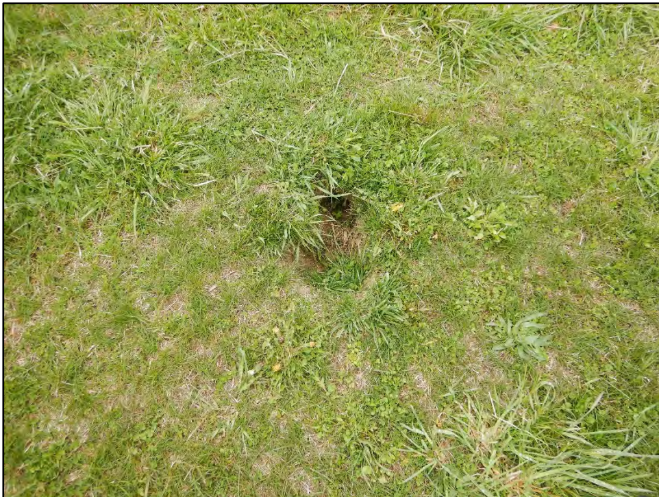
Figure 18: Photo taken on 4/20/21 showing an animal burrow on the dam crest.
