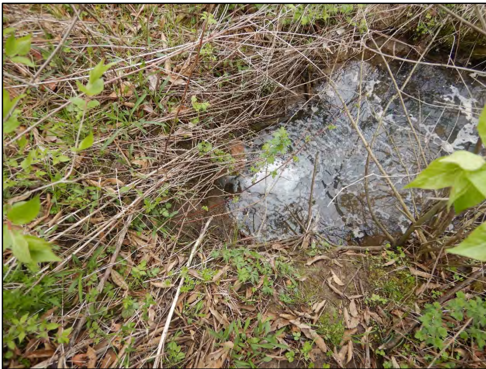
Figure 52: Photo taken on 4/20/21 the 6" CMP outlet with minor scour hole.
