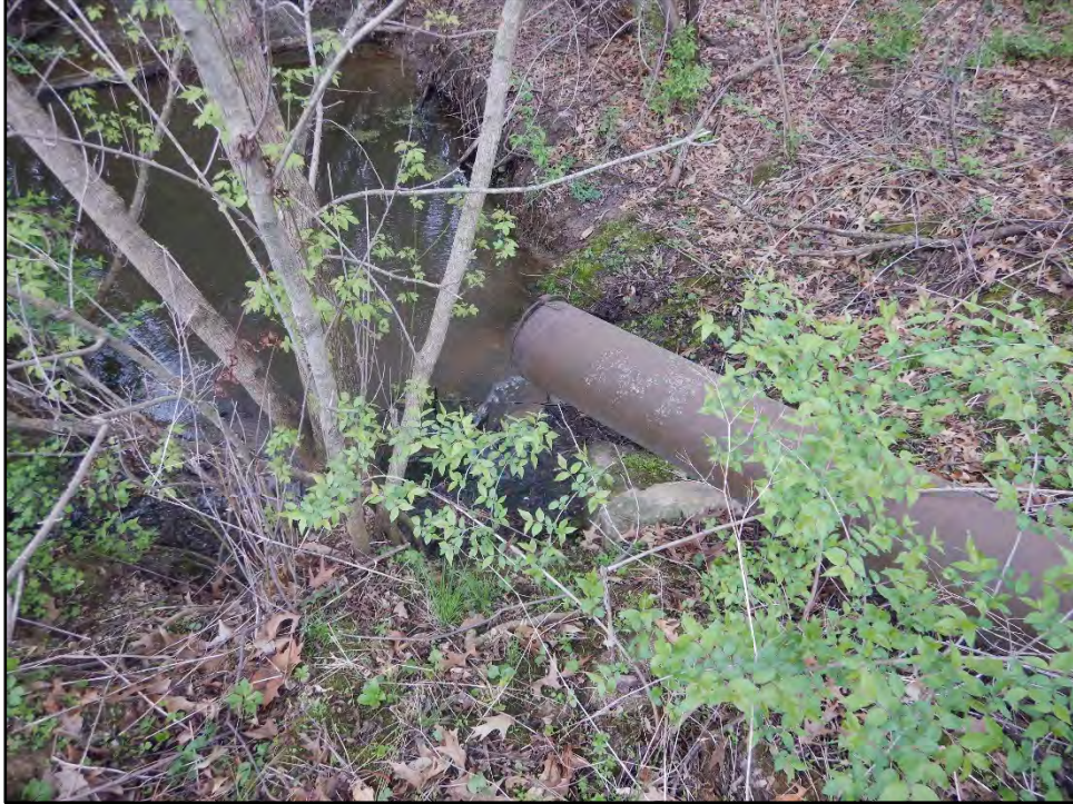
Figure 25: Photo taken on 4/20/21 showing the principal spillway outlet with rodent guard and small scour hole.
