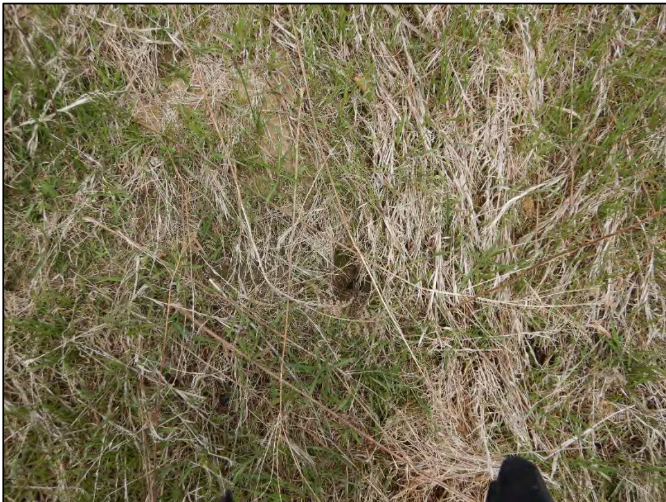
Figure 16: Photo taken on 4/20/21 showing rodent burrow on downstream slope.
