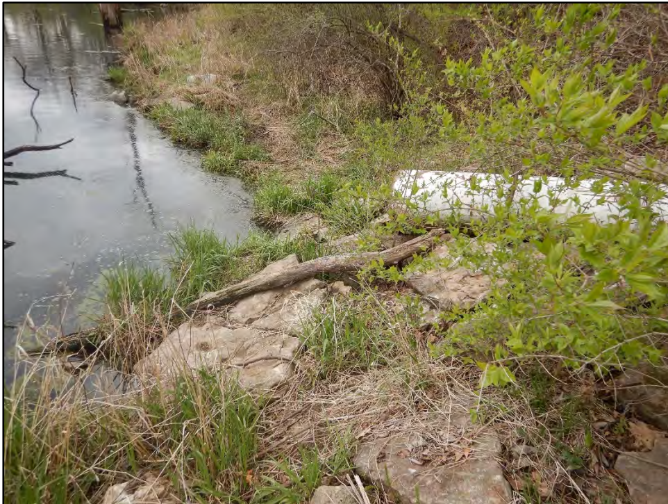
Figure 36: Photo taken on 4/20/21 showing the principal spillway outlet with rock riprap outlet and shoreline protection.
