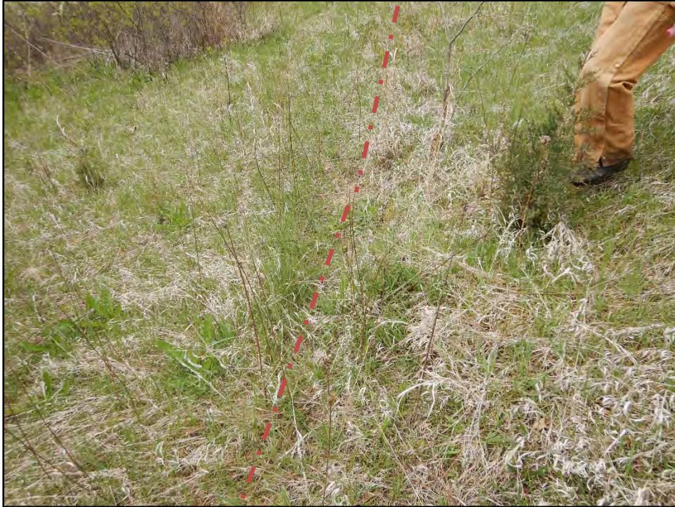
Figure 15: Photo taken on 4/20/21 showing signs of possible microslide on downstream slope signified by small bare grass line approximately 2/3 rd s up the embankment
