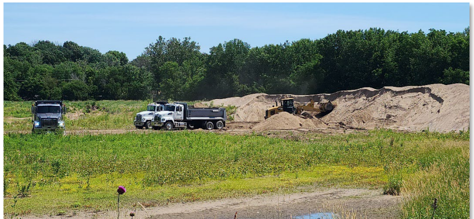
Photo 1 – USACE dredge sand from the Buffalo IA storage site being loaded for use in Waste Commission of Scott County’s new landfill cell construction project.
