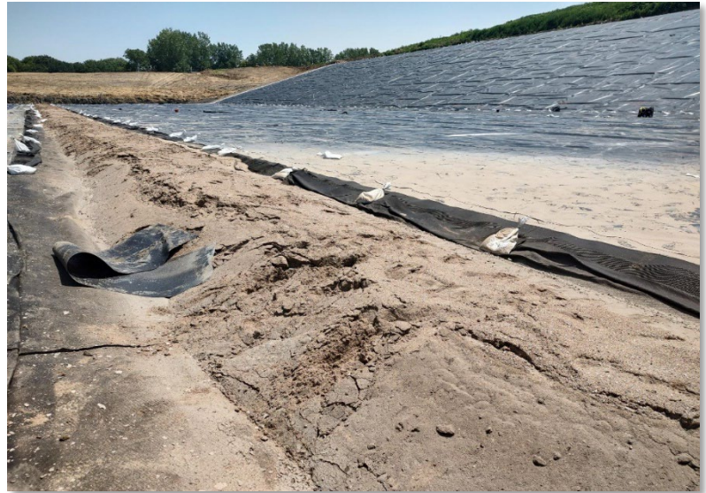
Photo 2 – Waste Commission of Scott County's new landfill cell construction showing placement of USACE dredge sand for the underdrain and leachate collection systems.
