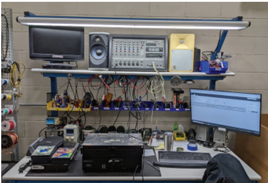
WCSC redesigned its electronics recycling center with facility electric upgrades and new equipment, such as this workbench.
