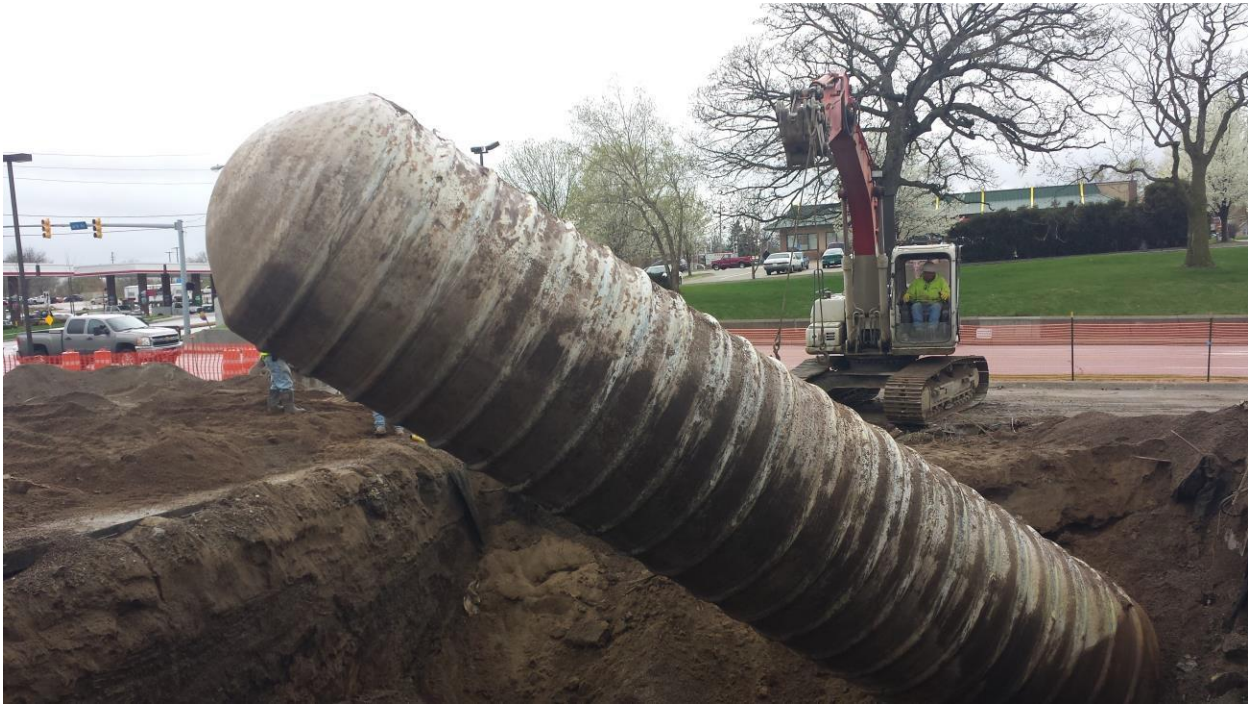
12000 gallon double wall Xerxes fiberglass tank removed in May 2014 at QuikTrip, 6 th and University Avenue, Des Moines.
