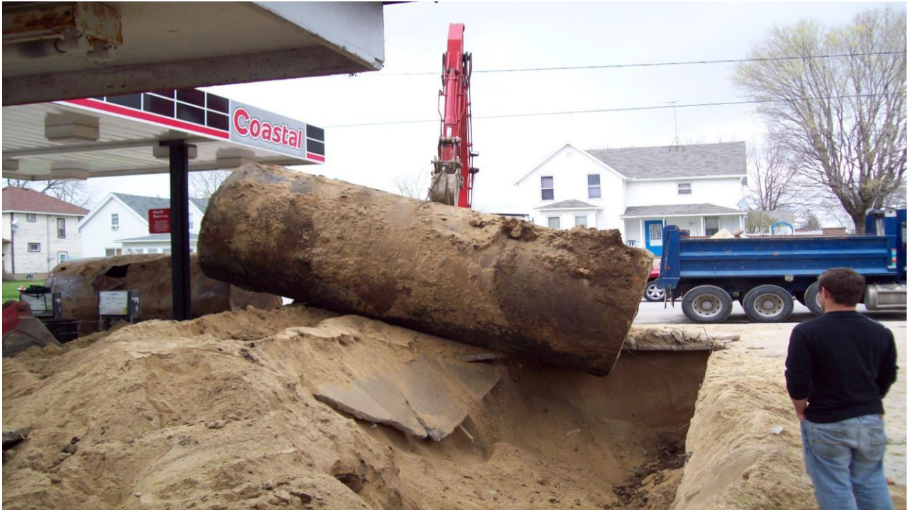
Tank removal in Waukon. Planning a tank removal must take into account overhead power lines and canopies that can present risks for removers. Please note, the person standing close to the excavation is not wearing safety equipment and the excavation is not barricaded.
