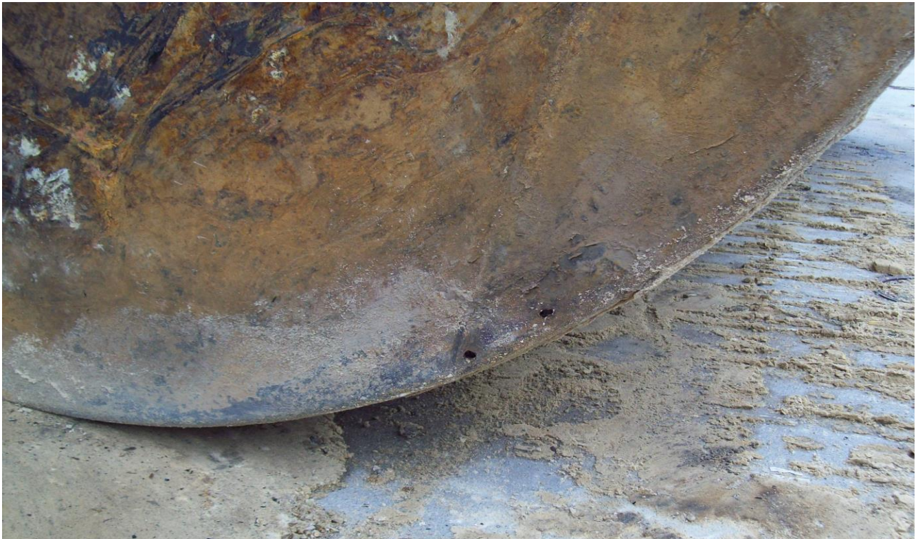
A documented release. This is the same tank as above. Note the two quarter-size perforations.
