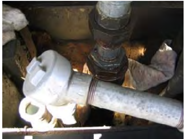
Not only do customers fill their vehicles directly over the cover of the monitoring well, a leak inside the dispenser travels right into the monitoring well (notice the rag around the pipe).
