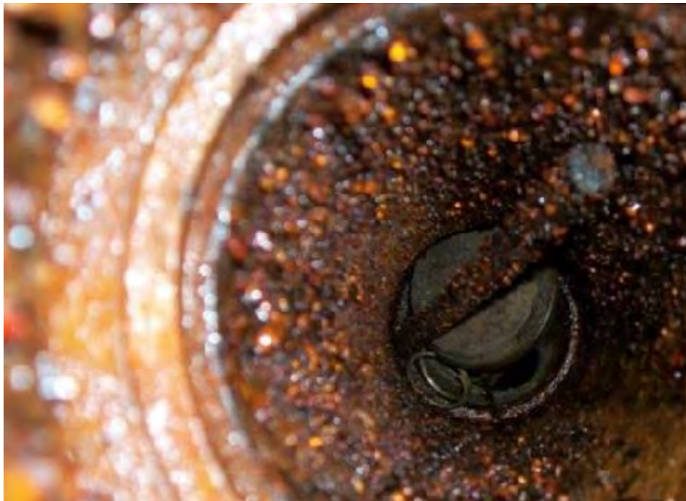
Dry Break on Stage 1 VRS pried opened and damaged by transporter, requiring replacement.
