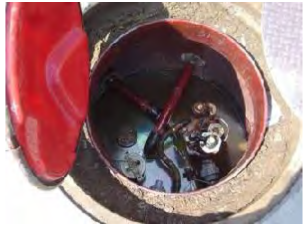
Photo 3: Same site with sheen on water in the STP sump
