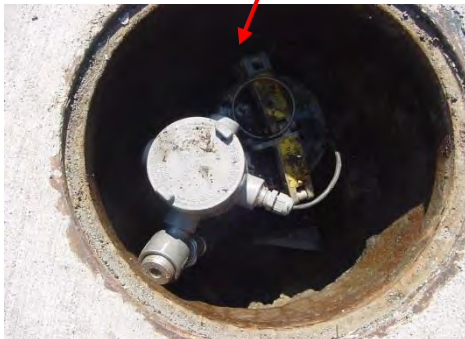
(ATG Access Manway)
