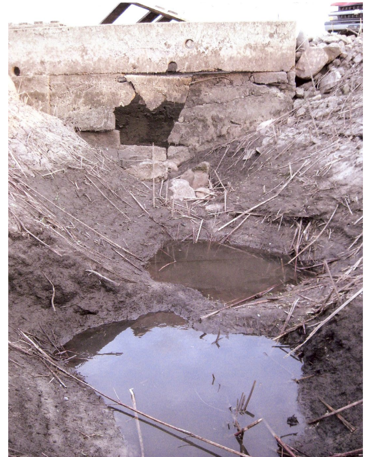
Broken Drainage System
