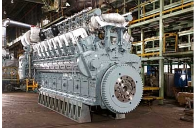
Older diesel engines may be cheaper to purchase, but may cost more when trying to meet air quality standards.
