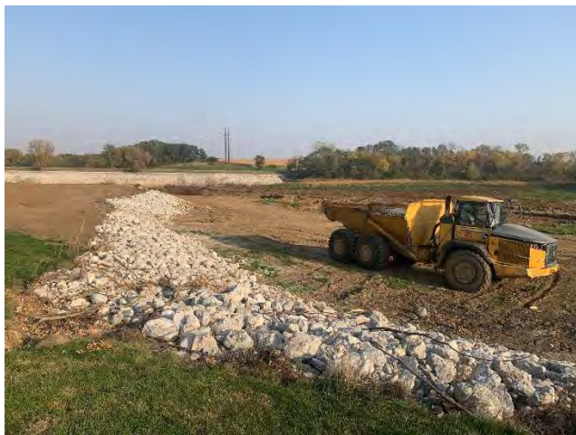
Shoreline stabilization along the banks of Lake of the Hills. Over 1000 feet of shoreline are being armored as a part of this project.
