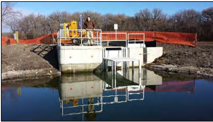
Pumping structure at the outlet of Marble Lake
