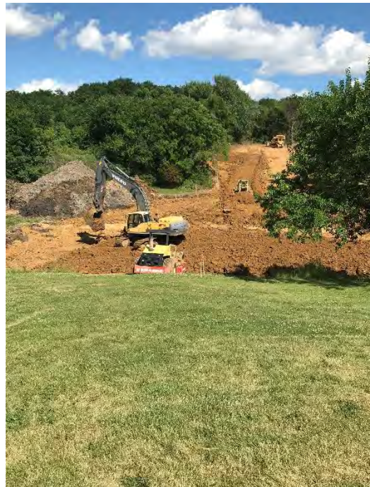
Construction at one of the watershed ponds constructed in the part as a part of the restoration efforts.
