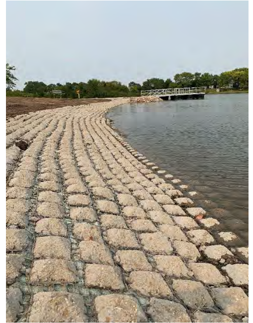
Flexamat (pictured here) was installed along the shoreline in 2020 to protect the lake from erosion and provide access to the water.
