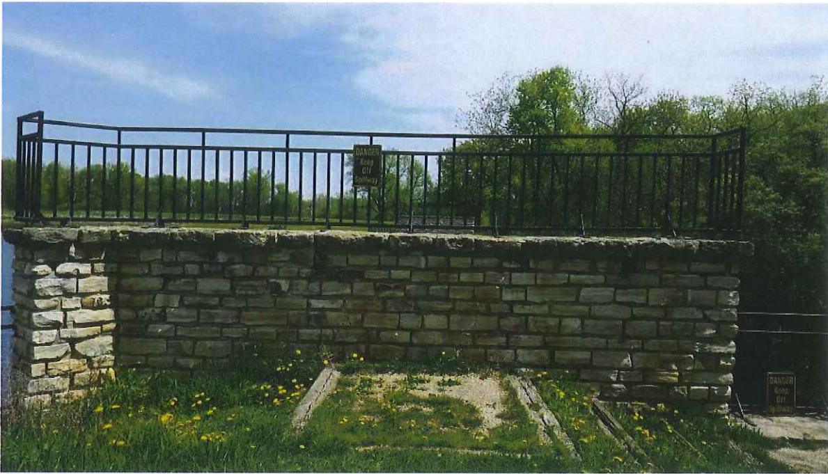
Warning signs at spillway
