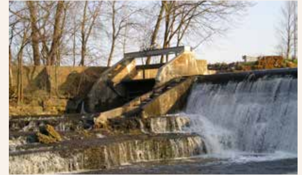
C3.A Quaker Mill Dam is one of the oldest remaining dams in Delaware County. Modification of the dam will preserve the base of the historic hydro electric plant.
