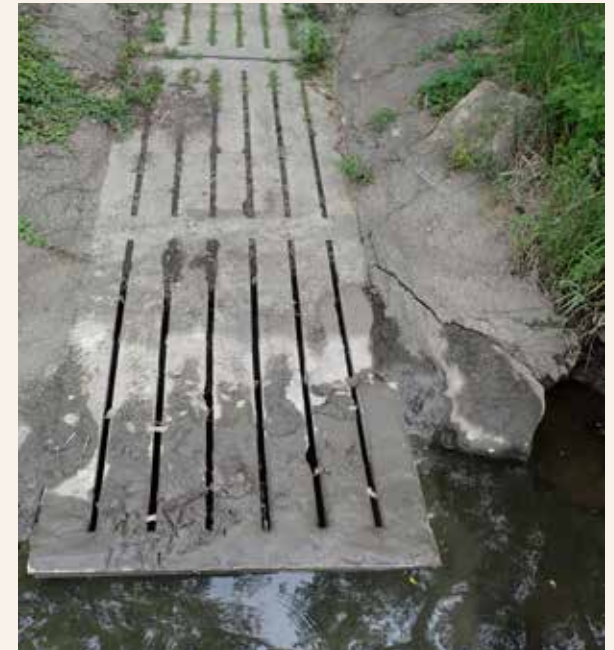
Figure 13 This hogslat-style launch at Tirrill Park has become damaged because of the way it was constructed and due to high water and streambank erosion.
